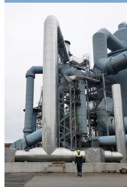
Waste heat recovery in Rönnskär.
