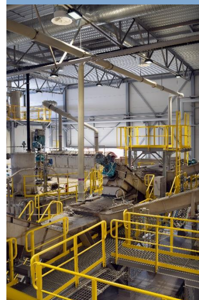
Plastic separation plant in Bergsöe.
