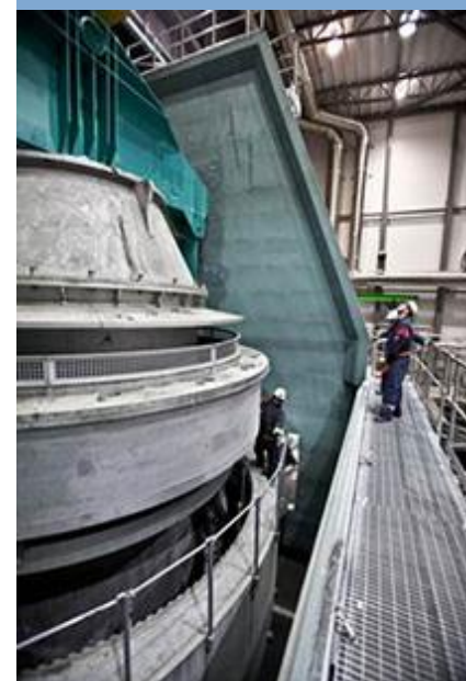
E-kaldo plant at Rönnskär
